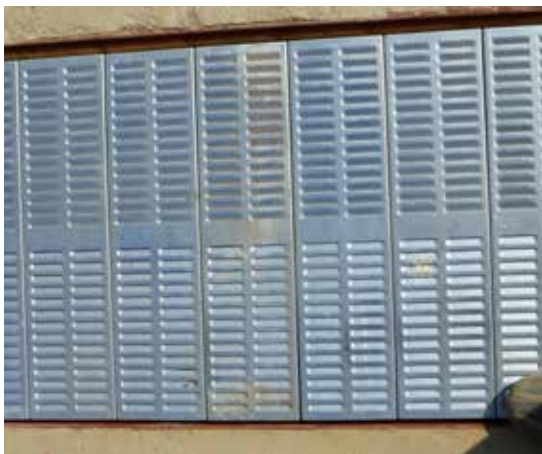
— Photo of floor aeration grids
